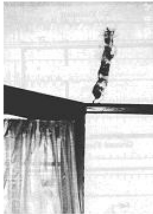
Figure 3.5: Damage on the southeast corner of south wall. (Tena-Colunga and Abrams 1992a).
