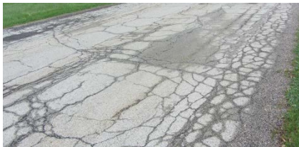
East Coral Road (Sections 1 and 2) before Overlay
