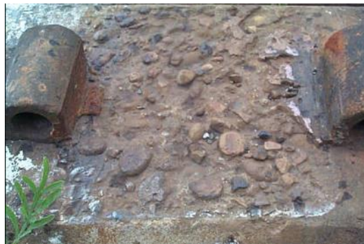
(b) Severe tangent RSD
