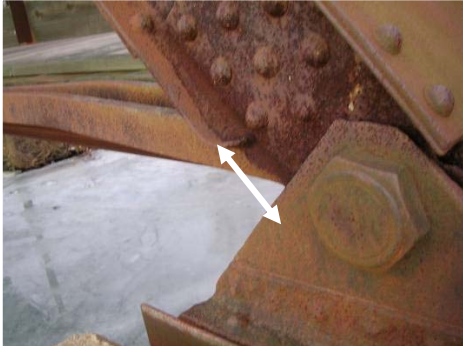
Figure 7.5. Corrosion of the bridge
