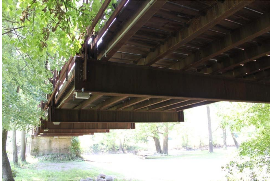
Figure 8.10. Sensors on the lower chords.
