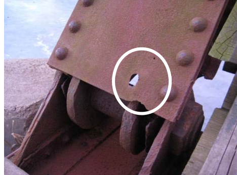
(a) Section loss and hole.
