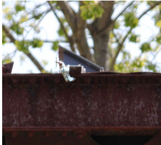
Figure 8.11. Sensor on the upper chords.
