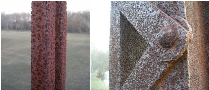
Figure 2.2. Corroded truss elements of the Mahomet Bridge.
