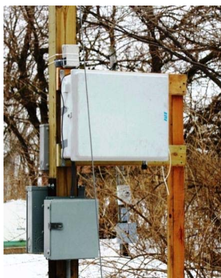
Figure 8.2. Base station enclosure.
