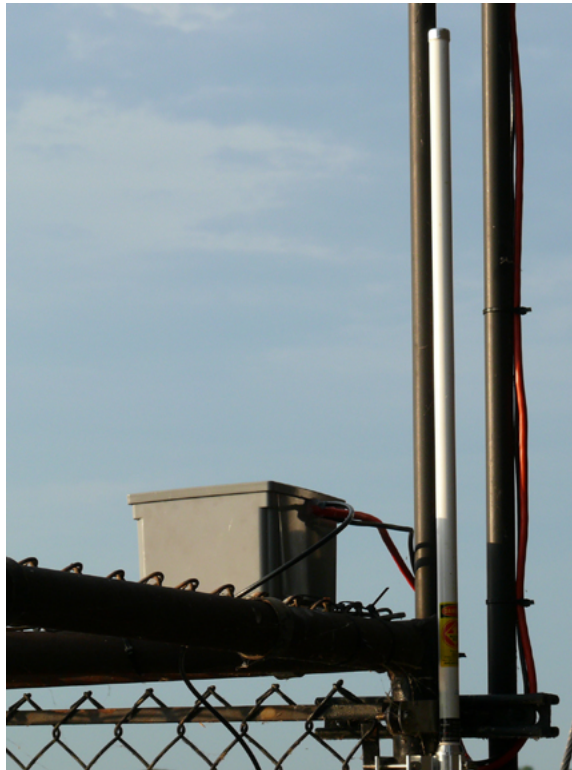
Figure 7.3: The gateway node installed outside the operator's house on the Government Bridge.
