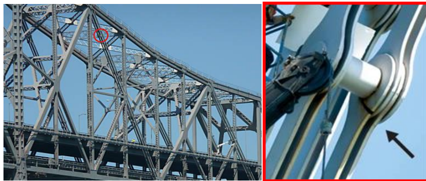
Figure 2.10. San Francisco-Oakland Bay Bridge and cracked eye bar by fatigue.
