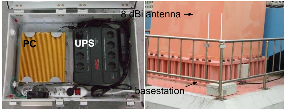
Figure 7.14. Basestation with PVC enclosure (left) and 8 dBi antenna for single-hop gateway node (right).
