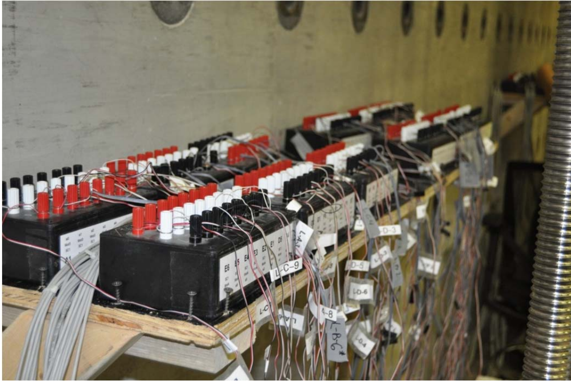
Figure B.17 Embedded and surface strain gage boxes - Pier 1
