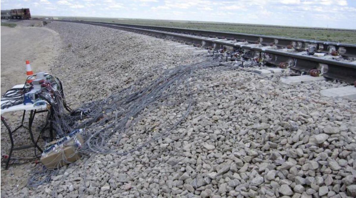
Figure E11: Instrumentation setup on the curved track (with freight consist approaching).
