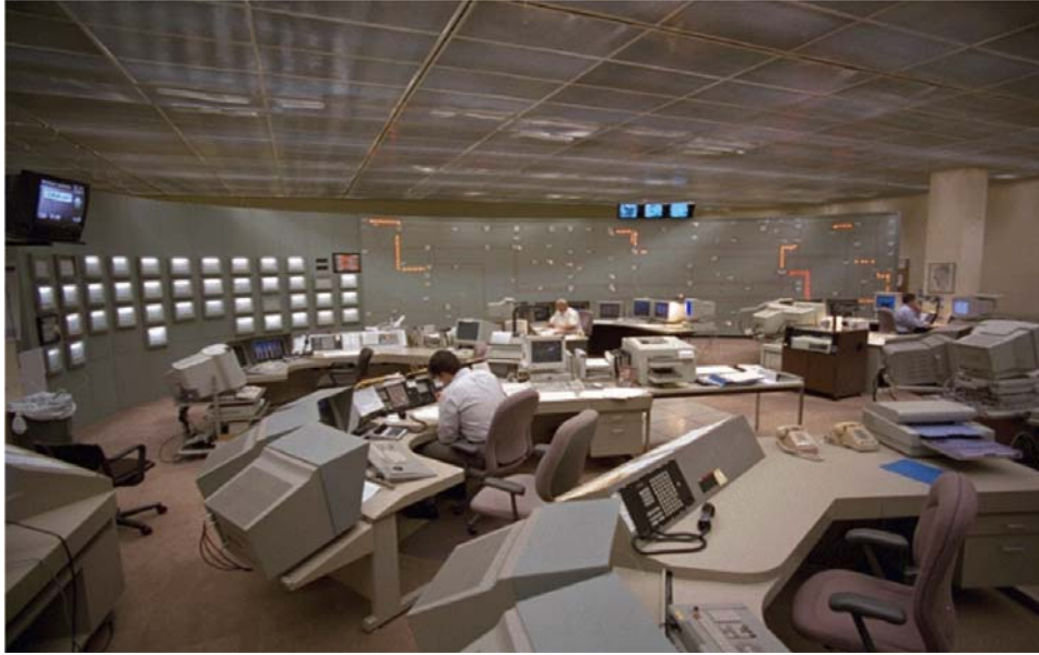
Figure 11: Commonwealth Edison control center in the late 1990s (Source: [73])
