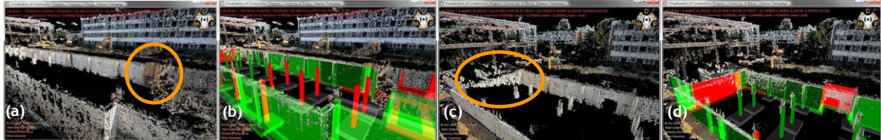
Figure 6.15. (a, b) False Positive – the formwork should not be detected as evidence of progress; (c, d) Missed Positive (False Negative) – the wall should be detected for progress though it is severely occluded.
