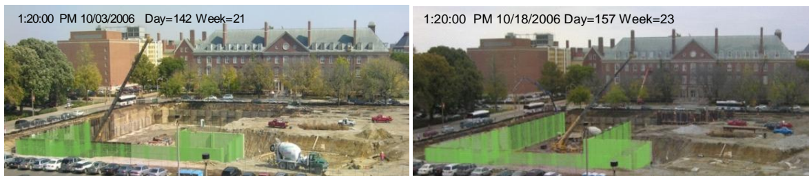
Figure 15. Two snapshots of the 4D model overlaid on time lapsed photographs during the simulated construction, UIUC College of Business Instructional Facility.
