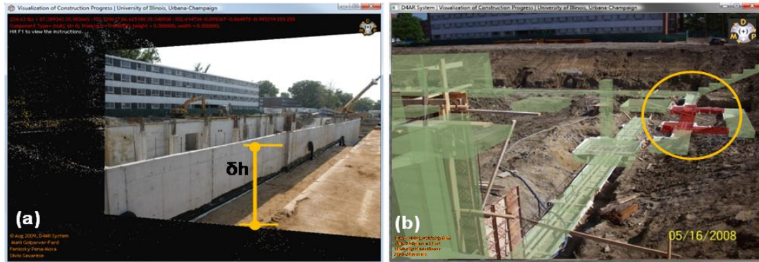
Figure 4.15. (a) Illustration of how trench depth can be measured; (b) Visualization of the foundation work. The section that needs to be formed for concrete placement is color-coded in red.
