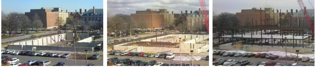
Figure 16. The time-lapsed progress photographs of college of Business Instructional Facility taken form a fixed camera installed on the site.
