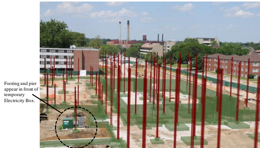
Figure 10. As-built model superimposed over the progress photograph. Student Dining and Residence Hall construction project in Champaign, IL. Images used are courtesy of Turner Construction (Used by permission).
