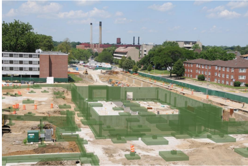
Figure 3.12. The alignment of the Student Dining and Residence Hall construction project 3D model with one of the construction progress images using Golparvar-Fard et al. (2009a) approach. As shown some of the foundations and foundation short walls as well as piers that are not yet constructed, are superimposed over the image. Photograph courtesy of Turner Construction Company; Champaign, IL; used by permission.
