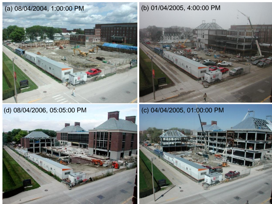
Figure 2.2. Progress images from a construction site time-lapse photography camera clockwise from 08/04/2004 to 08/04/2006 (Photograph subject: Institute of Genomics Biology, UIUC; Source: Information, Technology & Communication Services, College of ACES, UIUC).
