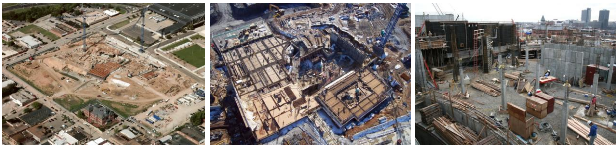
Figure 25. The Kauffman Center of Performing Arts images; The top image demonstrates the site from an Aerial point of view while the lower images from left to right are taken from a tower crane and from an interesting point of view using a regular digital camera.
