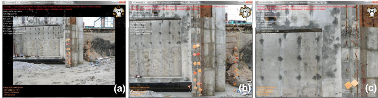
Figure 4.14. Illustration of interactive zooming. Capturing high resolution image along with the implemented interactive zooming allow the quality of the finished surface to be studied remotely. In addition safety issues (in this case rebar with no caps) could easily be observed from a very close range.
