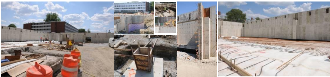
Figure 4. A Subset of daily progress photographs taken on Student Dining Construction Project. Photos Taken on 7/1/2008. Images courtesy of Turner Construction Co., used by permission.
