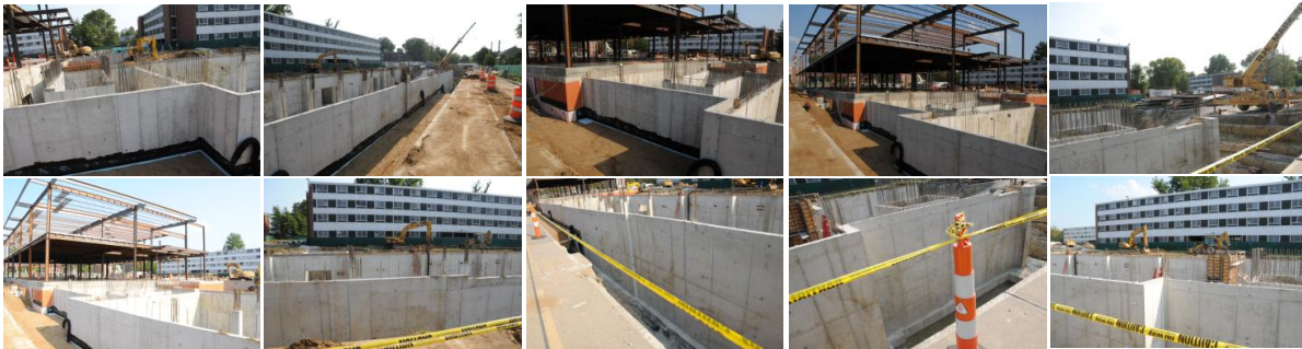
Figure 4.3. A subset of ten images represented from the 160 image set captured by the field engineer while monitoring the Ikenberry Residence Hall project on a walkthrough along the sidewalk. Images collected on 8/27/08 courtesy of Turner Construction; used by permission.
