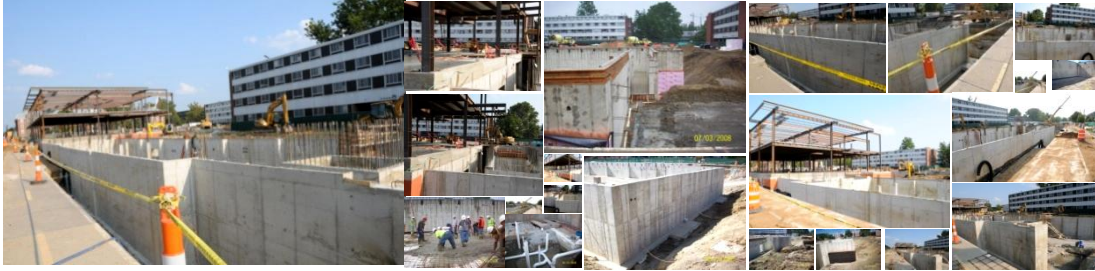
Figure 12. A Subset of daily progress photographs taken on Residence Hall-A Project. Photos Taken on 07/1/2008. Images courtesy of Turner Construction Co., used by permission.
