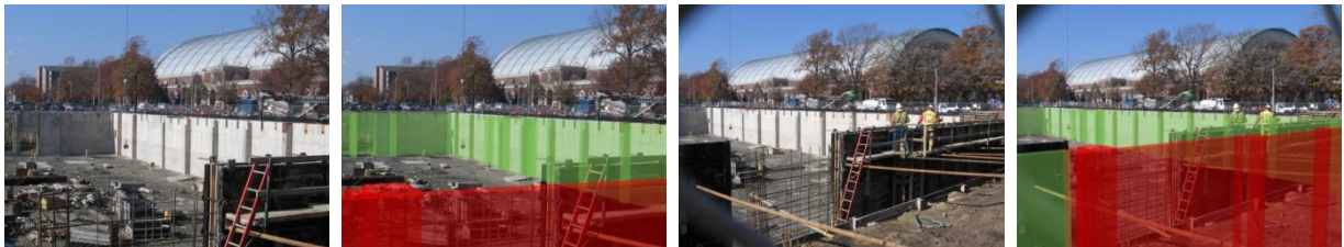
Figure 21. Randomly taken photograph of the construction site and the superimposed photograph representing progress status: From Left to Right: First two photographs: 11-07-06, 10:00AM, Second Two photographs, 11-08-2007, 11:20AM, UIUC College of Business Instructional Facility.
