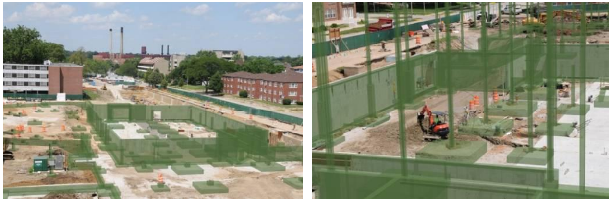
Figure 8. Snapshots of the 4D model superimposed over site images visualizing basement construction components as well as steel columns. (Images are courtesy of Turner Construction Co., used by permission).
