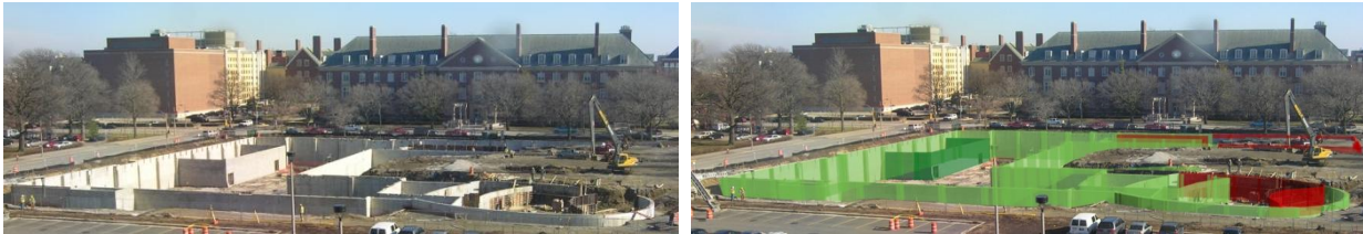
Figure 19. Time-lapsed photograph of the construction site and the superimposed photograph representing progress status, 01-03-2007, 12:35PM, UIUC College of Business Instructional Facility.
