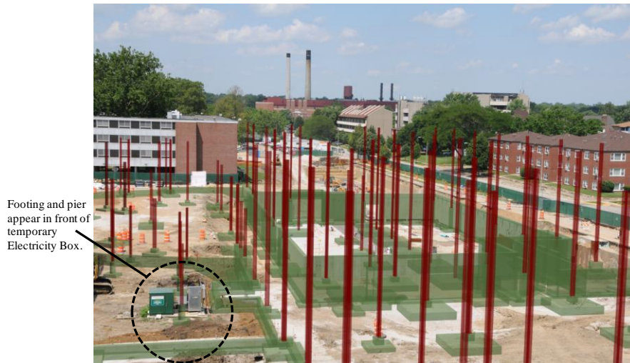
Figure 3.20. As-built model superimposed over the progress photograph. Student Dining and Residence Hall construction project in Champaign, IL. Photograph courtesy of Turner Construction Company; Champaign, IL; used by permission.
