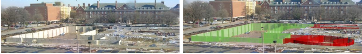
Figure 18. Time-lapsed photograph of the construction site and the superimposed photograph representing progress status, 12-02-2006, 1:13PM, UIUC College of Business Instructional Facility.
