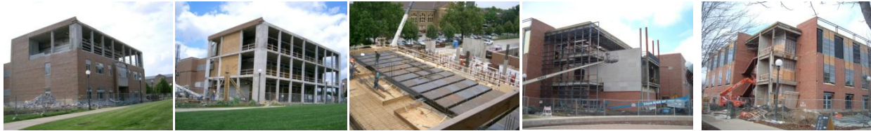
Figure 27. Photographs taken from demolition phases to the end of the construction phase from different angles and point-of-views, Micro and Nanotechnology Lab Extension Project
