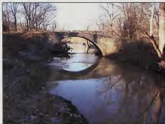
Figure 30 Fountain Creek Stone Bridge, located just west of Waterloo, Illinois, on Route 156, was built from locally quarried limestone in 1849. (Photograph by Samuel V. Panno.)
