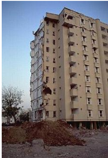
Figure 6. Progressive collapse of left side of building (SED, 2011)
