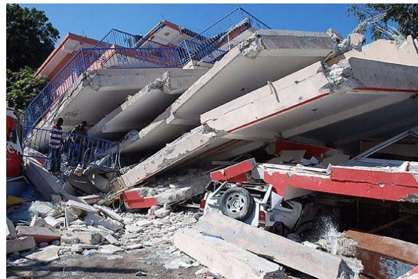
(b) 2010 Haiti Earthquake (Lorant, 2010)
