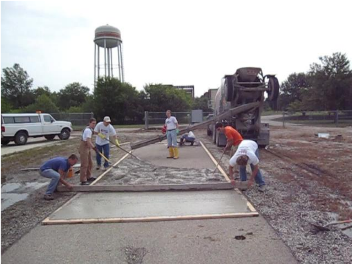
Figure A-4 Photograph of the construction of the trial section using rakes to spread the concrete and a wood screed for finishing.
