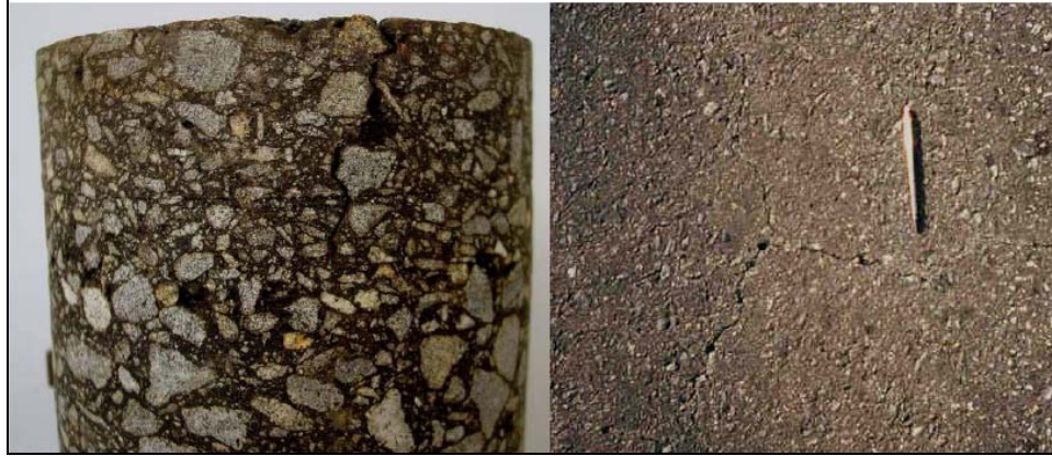
Figure 2.4 Observed top-down cracking in field (after Uhlmeyer et al., 2000)
