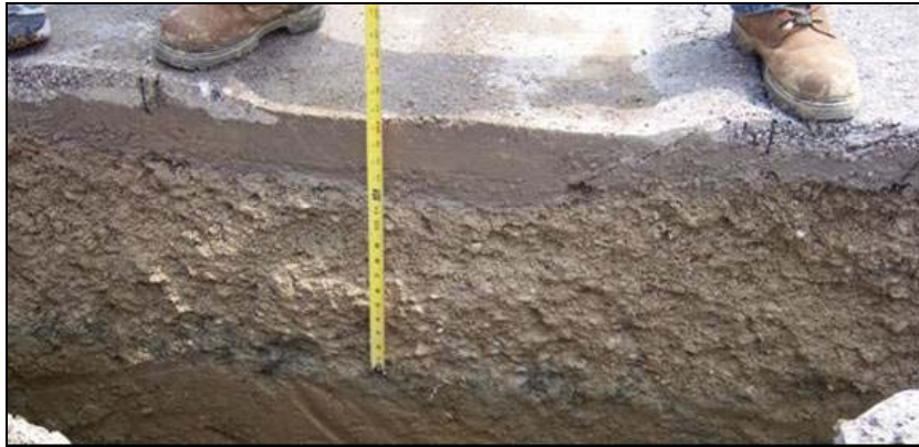
Figure 2.3 Observed shear failure in asphalt layer caused by rutting in granular base layer and subgrade (after Al-Qadi et al. 2007)
