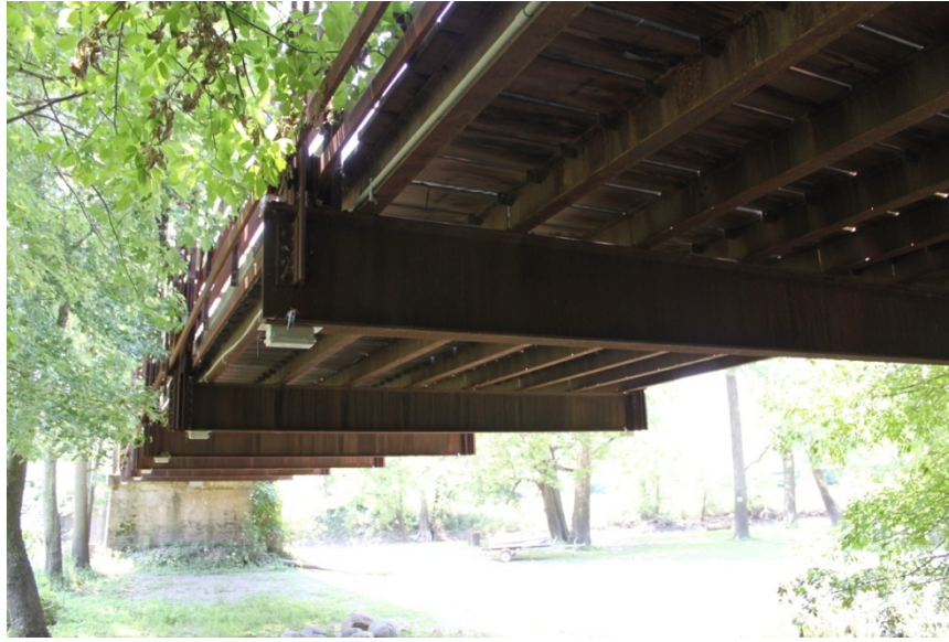
Figure 8.10. Sensors on the lower chords.
