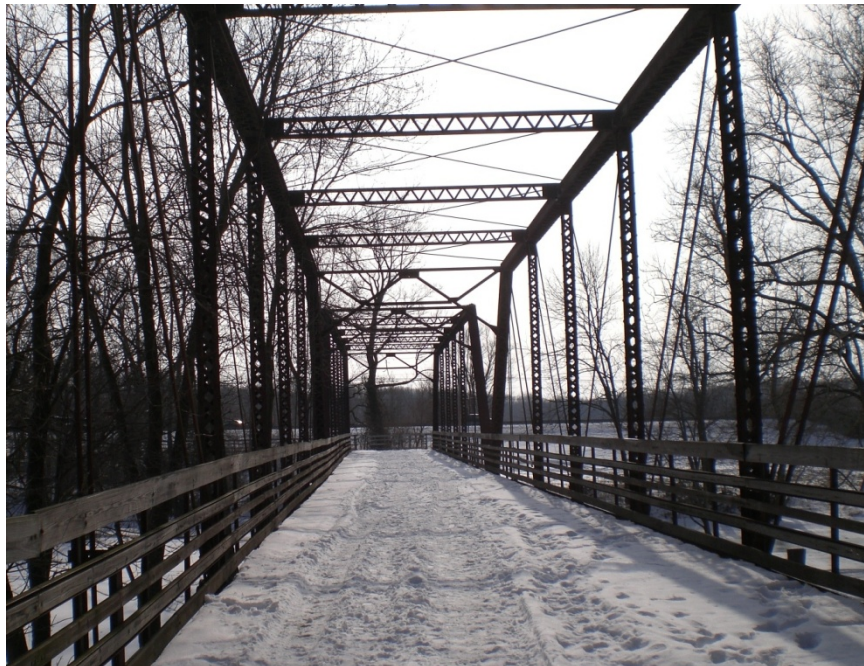
(a) Mahomet bridge on January 14, 2010
