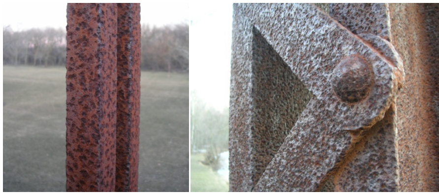
Figure 2.2. Corroded truss elements of the Mahomet Bridge.
