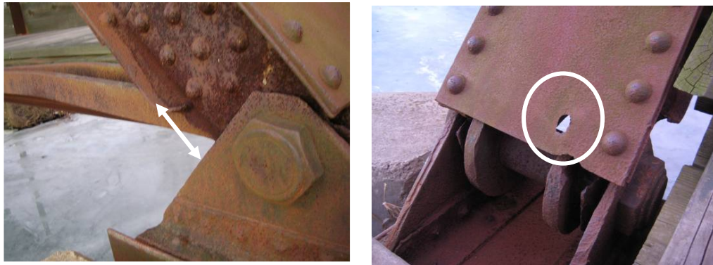
(a) Section loss and hole.
