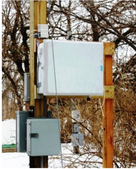
Figure 8.2. Base station enclosure.
