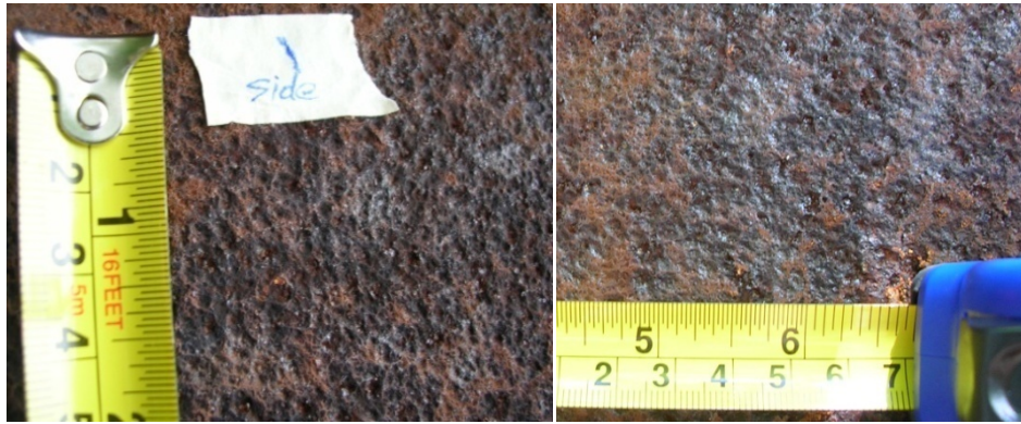
(a) Section 1 in 2008 (left) and in 2010 (right)
