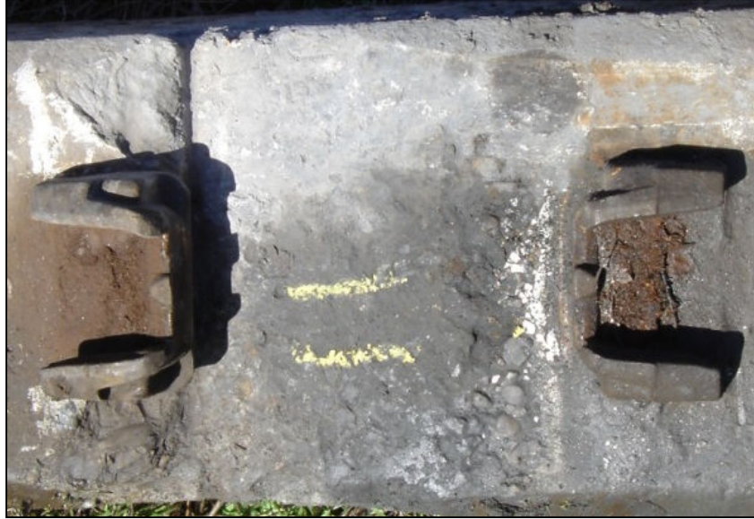
Figure 2.7 Example of concrete-tie rail seat deterioration (RSD)
