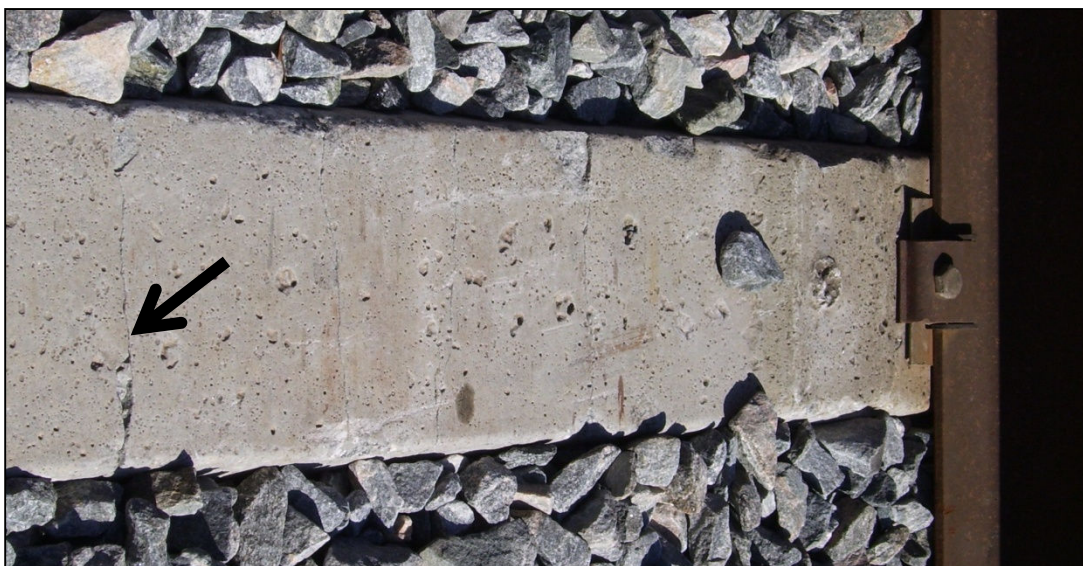
Figure 2.2 Example of a center-negative, flexural crack, suggesting a center-bound condition
