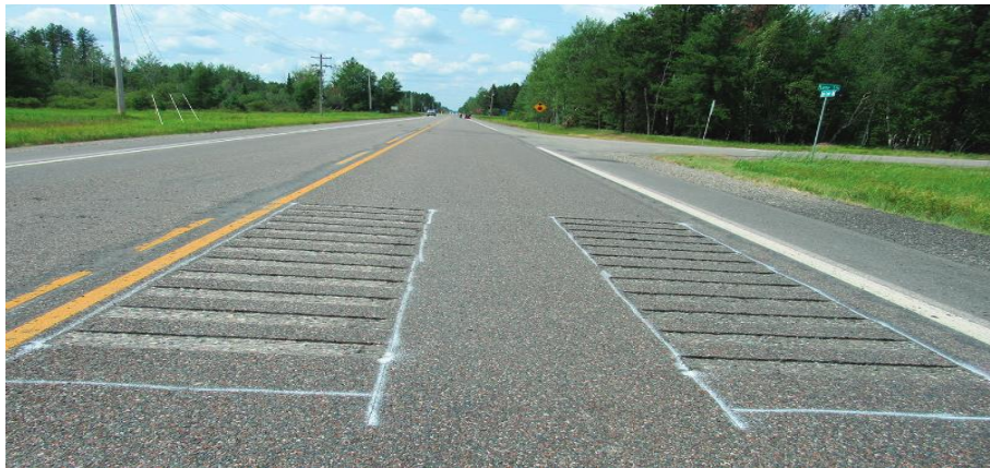
Figure 93. Photo. Wheel path transverse rumble strip.
