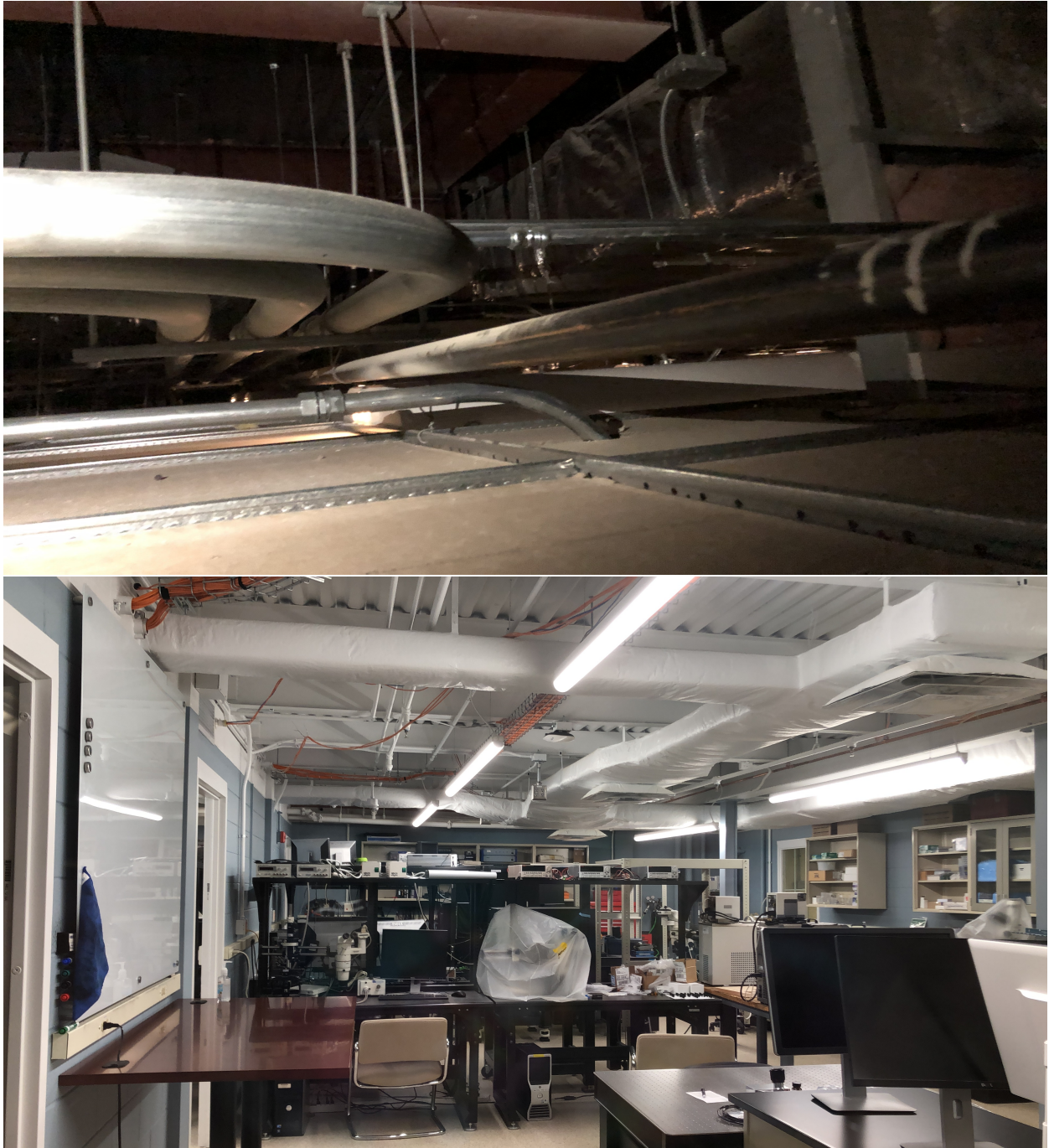
Figure 4.3: Mechanical Systems Above a Suspended Ceiling (upper photo) and Below an Open Ceiling (lower photo).
