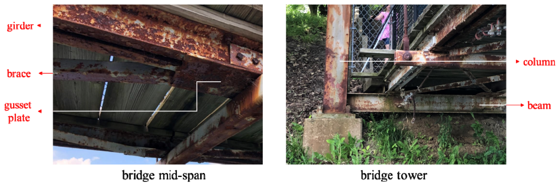
Figure 7.12 Corrosion of the bridge in mid-span and bridge tower.
