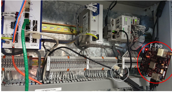
Fig. 5: F-Pro integration into EPIC Testbed [18]. On the right side, we highlighted one of the F-Pro devices connected to a switch in the generation segment (GSW2), with the two highlighted cables in bump-in-the-wire manner.
