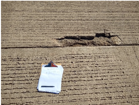
c) Severe joint damage in DL and Shoulder - Approach (3299+68 WB)
