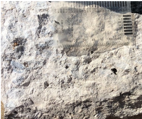
e) Concrete shows entrapped air
