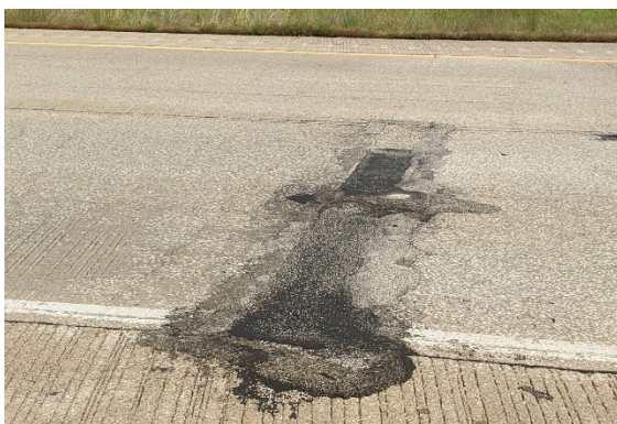
e) HMA Patch over punch-out (464+88 EB)
