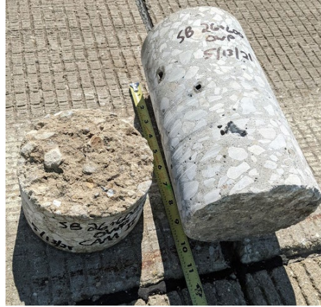
b) US 67 SB 26+600 outer wheel path core (CAM II potentially eroded surface on left)
