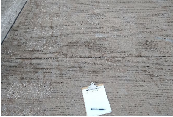
a) Durability cracking in the Outer Shoulder (24+594 NB)
