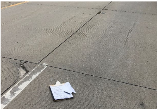
c) Corner failure in PL approach and reflector damage (1+715 EB)
