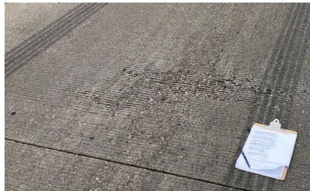
d) Ravelling on concrete surface in DL (180+90 NB)
