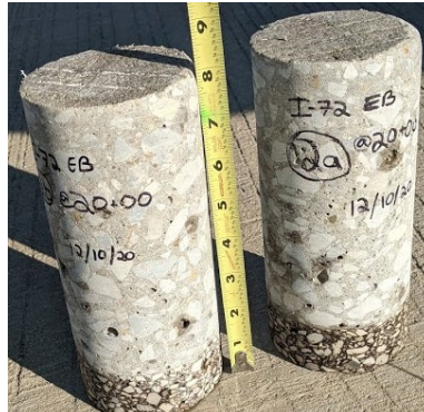
Outer wheel path (approach joint): NOT over longitudinal crack
