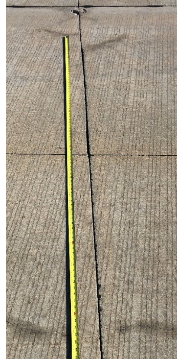
b) Distance between long. cracks at the trans. jt. (approx. 7.5-8 ft)
