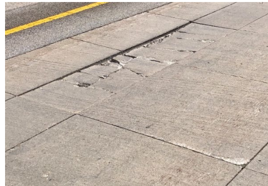
f) Additional Long. jt. causing cracking and punchout (similar to CRCP)
