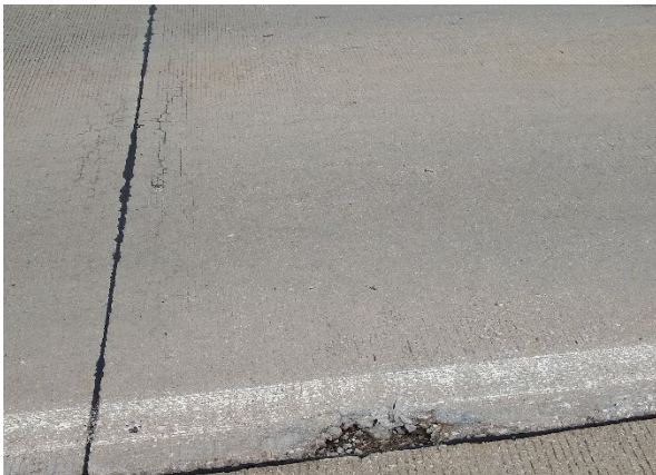
e) Longitudinal joint spalling and transverse micro-cracking along joint (26+056 SB)
