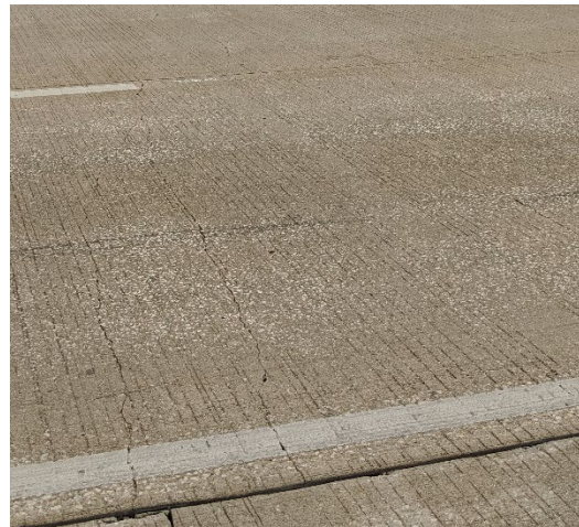
f) Y-cracking and complex Y-cracking (304+00 WB)
