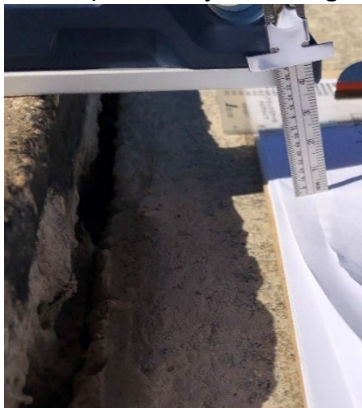
e) Long. faulting along OWP DL long. jt. (8+96 SB): ~1.8 in. (46 mm)
