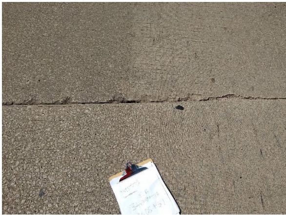
c) Joint spalling with corner spalling along Approach joint in DL (3405+51)
