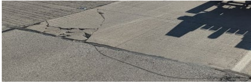
Figure 224. Photo. Distress photos of shattered slab in I-72 (72G92) EB.
