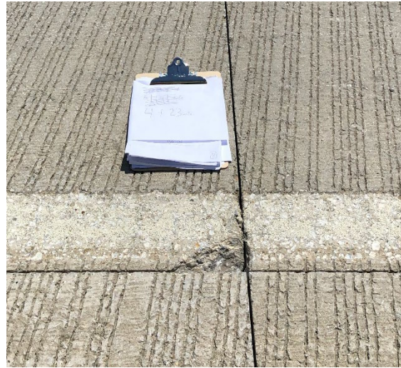
b) Milling of rumble strips effect on approach joint causing corner distress
