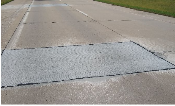
a) New FDR performing well in DL; corner failure in PL (28+660 SB)
