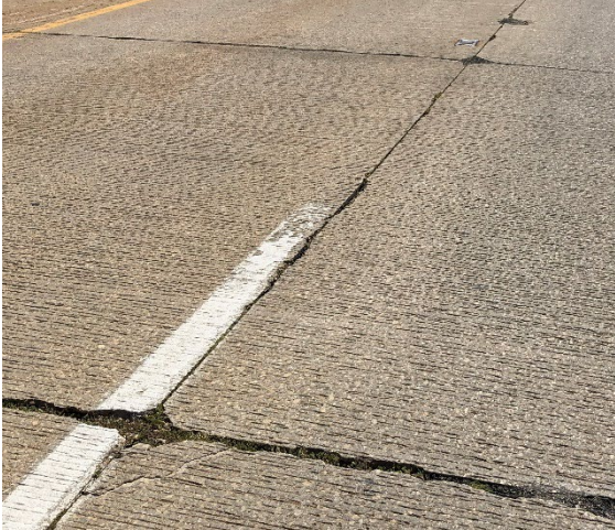
a) Joint deterioration (989+50)
