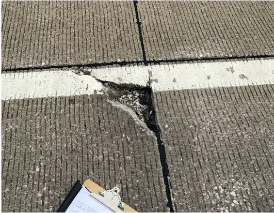
g) Corner failure with pop-out in DL between PL/DL (2+070 WB)
