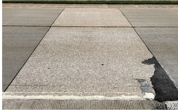
h) FDR with HMA patch and Longitudinal faulting (2+030 WB)
