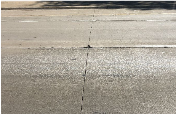
c) Corner distress and diamond grinding (234+47 SB)
