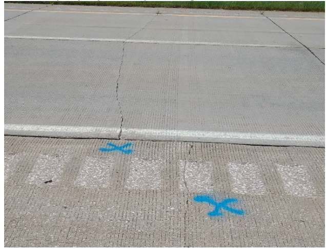
d) Transverse crack with spalling and faulting (26+498 SB)
