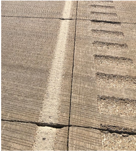
a) Milling of rumble strips effect on approach joint spalling
