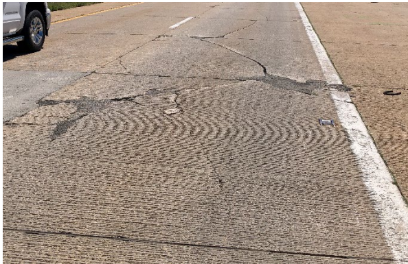
c) Shattered slabs in DL with some HMA patching (996+70)
