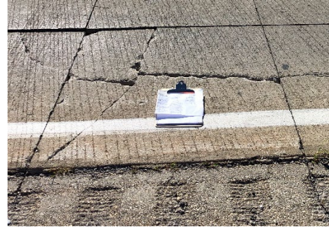
d) Shattered slab (2+64 SB)
