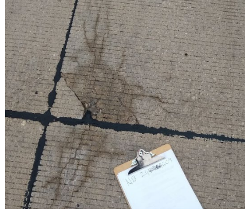
b) Corner distress or durability cracking in DL (24+609 NB)
