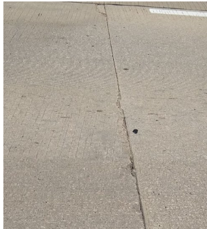
d) Joint spalling with corner spalling along Approach joint in DL (3405+51)
