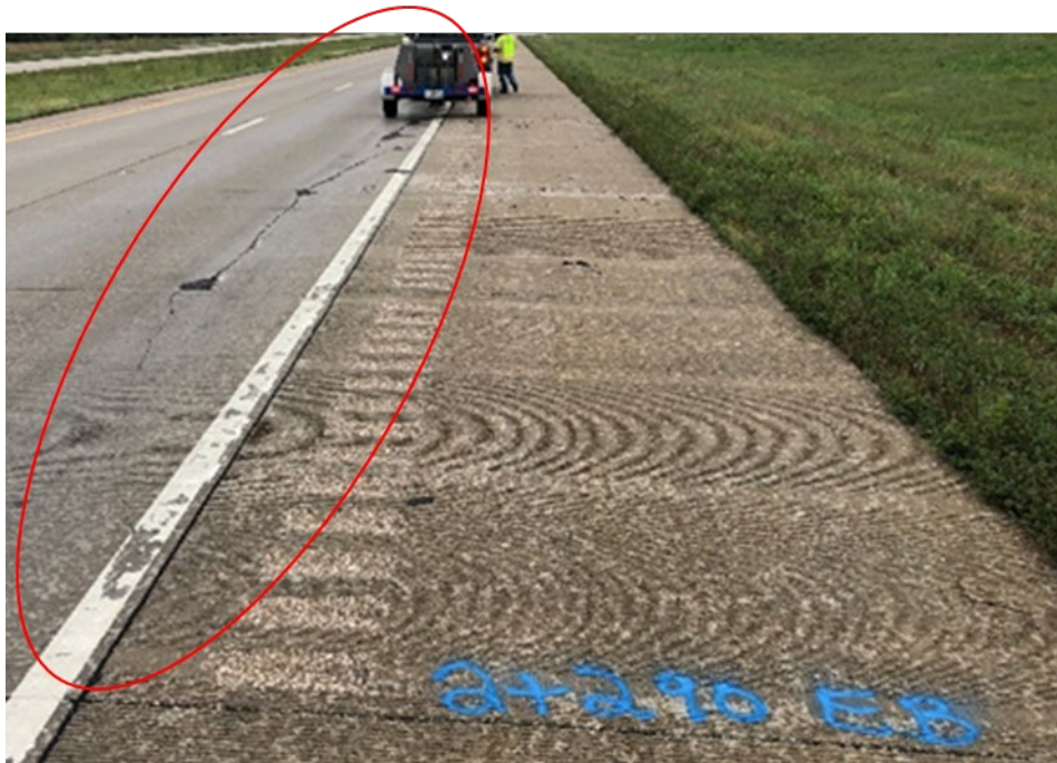
Figure S1. Photo. Loss of support beneath the concrete pavement on I-72 (92763).
