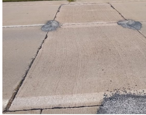
b) Old FDR with excessively wide joints and HMA or spray injection patching (28+615 SB)
