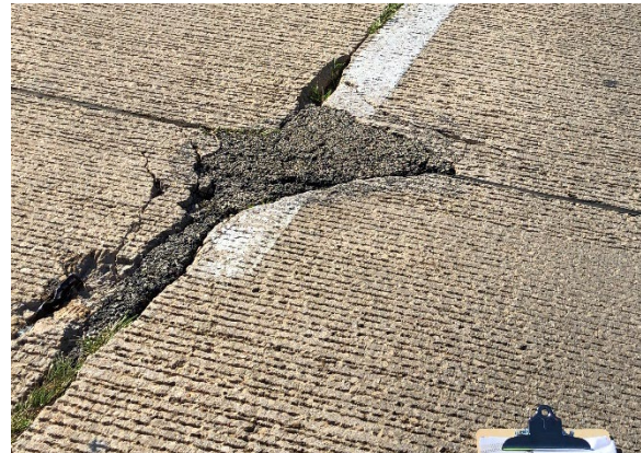
d) Long. jt. deterioration with HMA patch (901+00)
