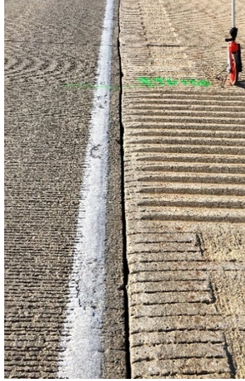
a) Lane-shoulder long. jt. (896+00)
