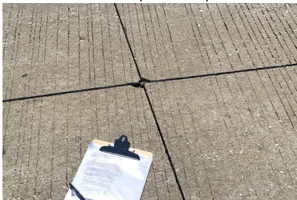
e) Minor corner spalling (150+45 to 149+00 SB)
