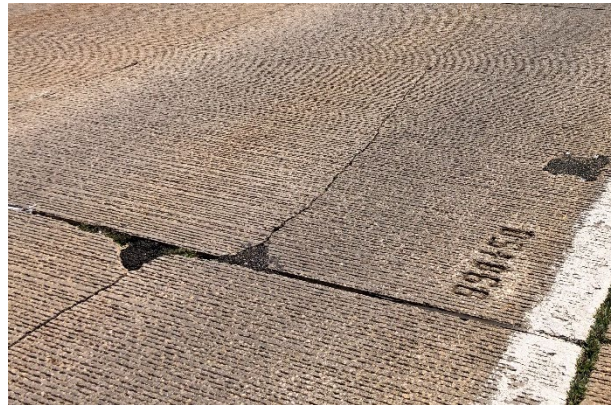
b) Mid-lane long. cracking in DL (998+50)
