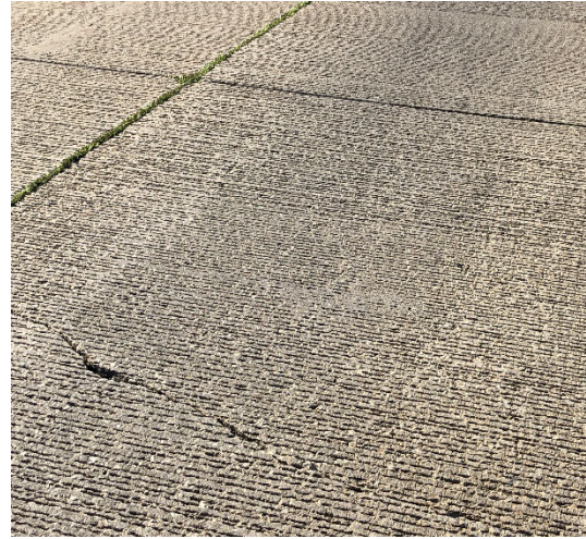
b) Trans. cracking and vegetation growth in long. jt. (897+60)
