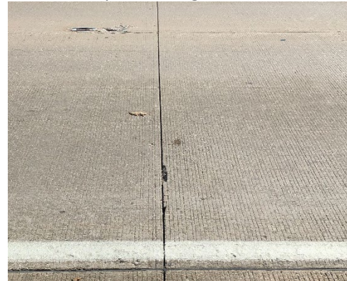
d) Transverse joint spalling (199+50 SB)
