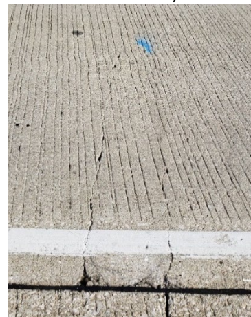
d) Y + Divided cracking (249+56 EB)
