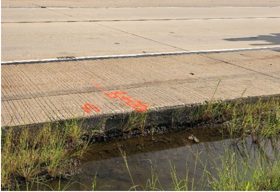
a) Free edge has pooling of water (8+00 EB)
