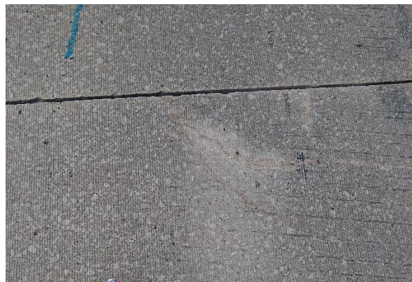
f) Surface cracking diamond ground (3407+46)
