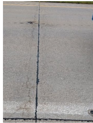
d) Durability cracking in the DL and PL with pop-out (26+016 NB)
