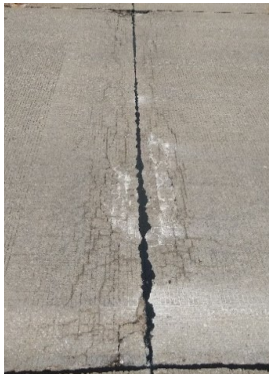
Figure 22. Photos. US 67 SB 23+839 distress at transverse joint.
