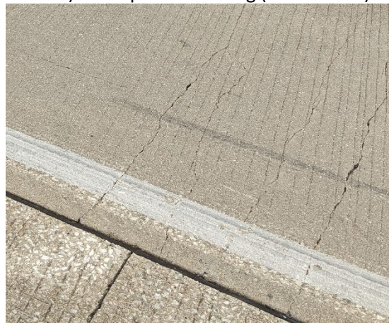
d) Y-cracking (409+96 WB)
