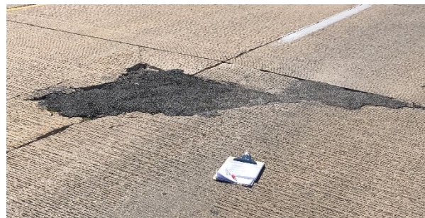
f) Corner break spanning DL and PL with HMA partial depth repair (903+00)
