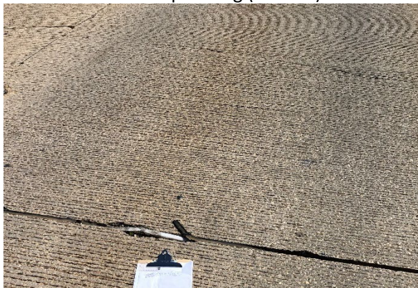
e) Mid-panel trans. cracking and jt. sealant damage (1001+15)
