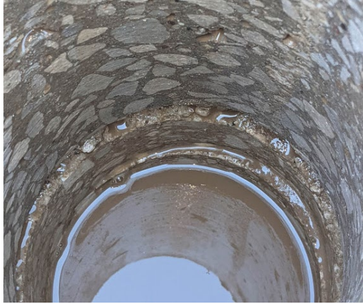
a) US 67 SB 26+600 outer wheel path coring hole
