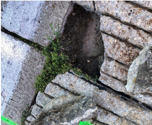
c) Corner crack and popout with fines slurry along lane-shoulder long. jt – leave slab in shoulder (898+00)
