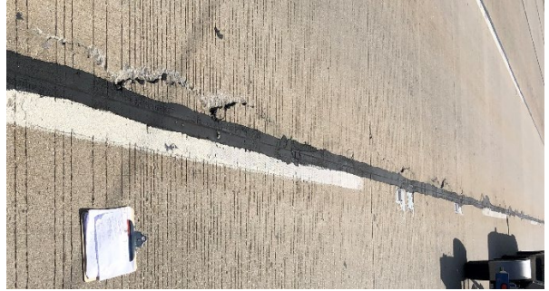
b) Severe long. cracking along long. jt between DL & PL (70+75 EB)
