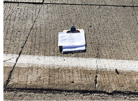
b) Trans. cracking (2+36 SB)
