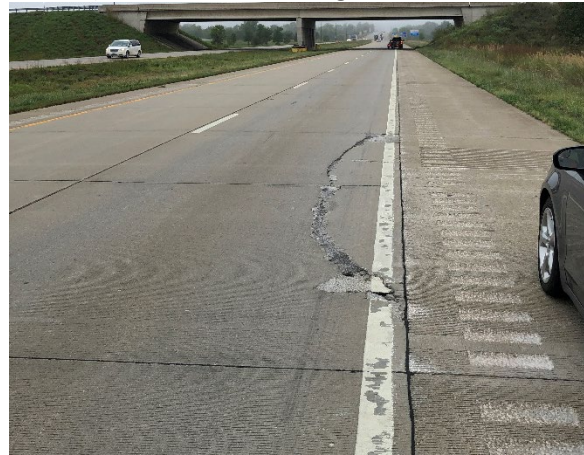
d) Edge failure due to lack of support (2+250 WB)
