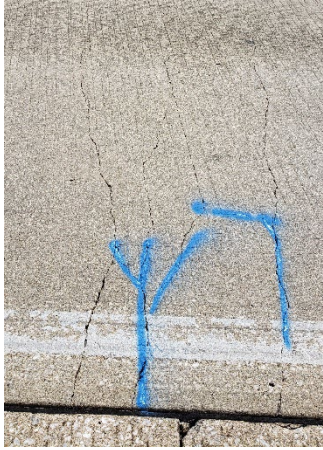
a) Complex Y-cracking (411+28 WB)
