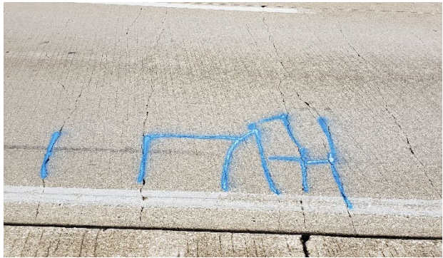
b) Complex Y-cracking (411+49 WB)
