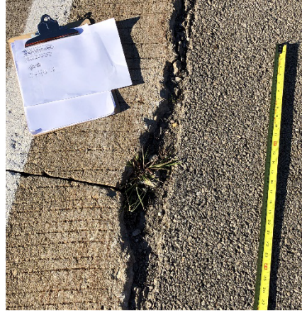
b) Lane/shoulder long. jt. degradation
