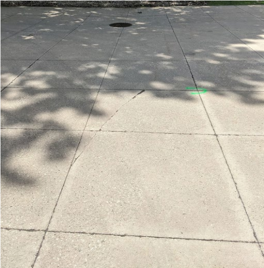
c) Diagonal cracking in northeast bay
