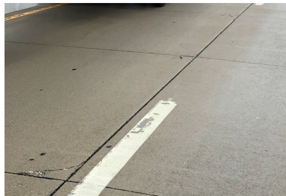
f) Corner distress in PL (Section EB-4)
