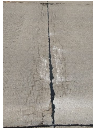
f) Severe ASR (23+839)
