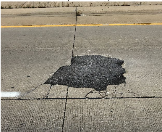
e) Corner break with HMA patch in PL on Approach and Leave (181+55 NB)
