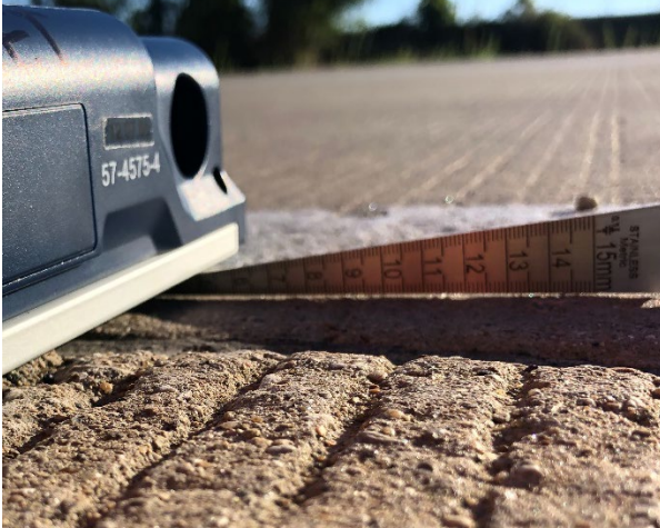
a) Long. joint faulting: Shoulder > DL (0.2 in.) – (277+82 to 276+00 SB)
