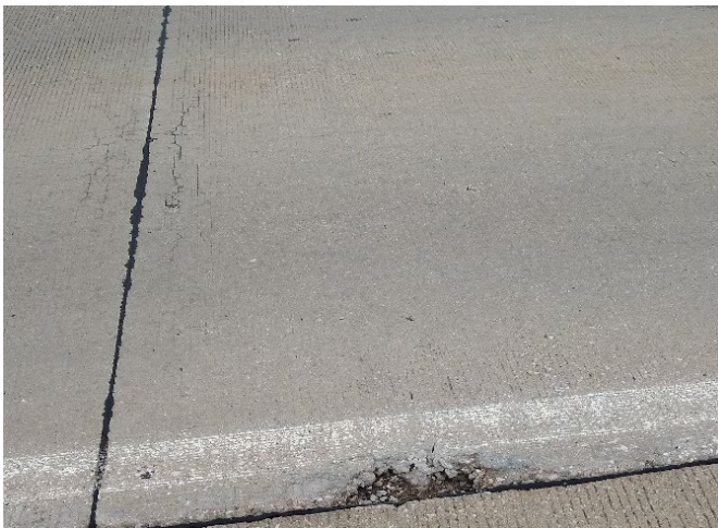
e) Longitudinal joint spalling and transverse joint deterioration (26+056 SB)
