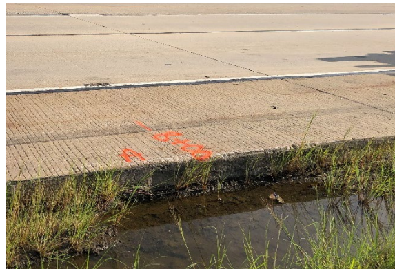
Figure 192. Photo. US 30 (62277) EB 8+00 core location #3 with pooling of water along free edge.
