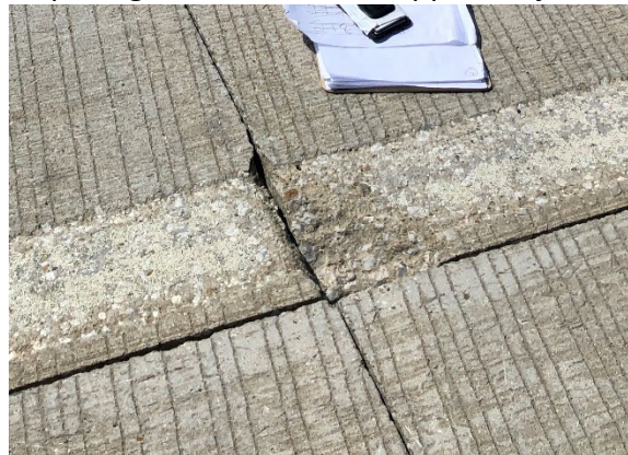
c) Milling of rumble strips effect on leave joint corner distress
