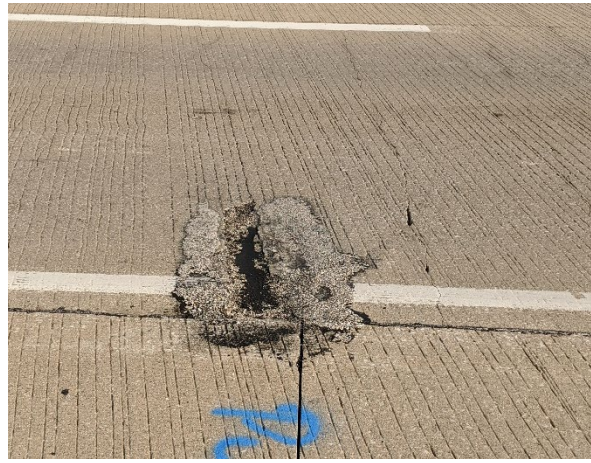
b) Punchout filled with HMA patch (247+35 EB)
