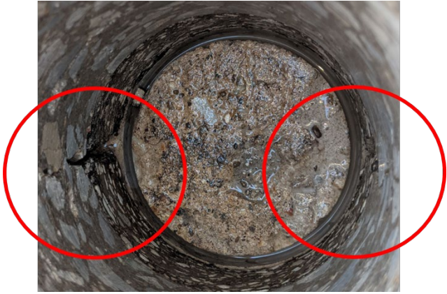
B. 14+02 EB OWP crack deterioration in HMA at transverse joint
