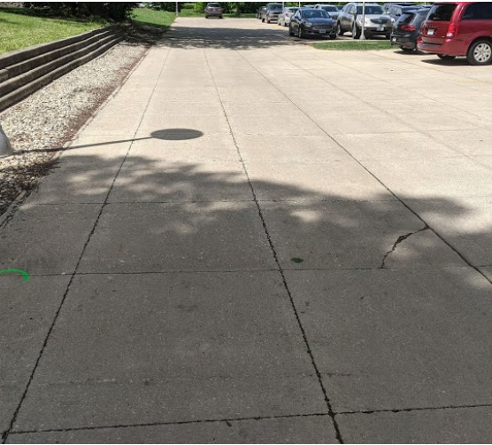
a) Corner break in southeast bay
