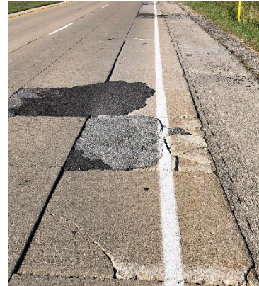
f) Typical observed failures in DL OWP
