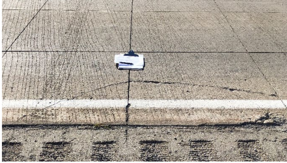
c) Slab cracking across three panels (L/S jt. edge)
