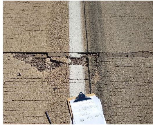
b) Corner failure, joint spalling and faulting in DL and Shoulder – Leave (3299+99 WB)
