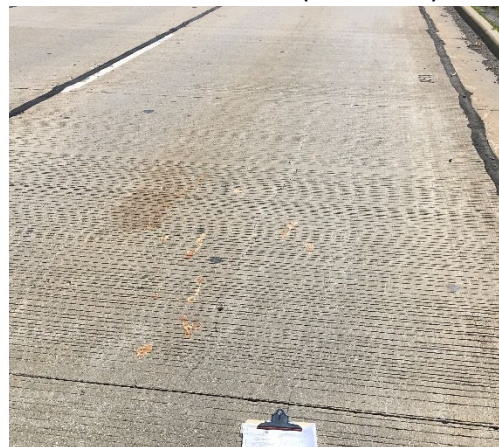
d) Long. cracking mid-slab spanning two panels (72+00 EB)
