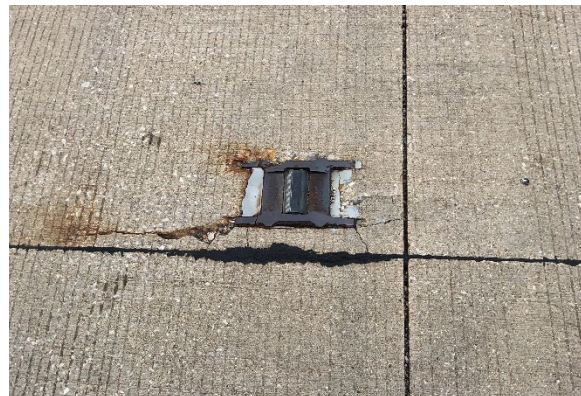
f) Distress from embedded raised pavement markers (multiple locations)
