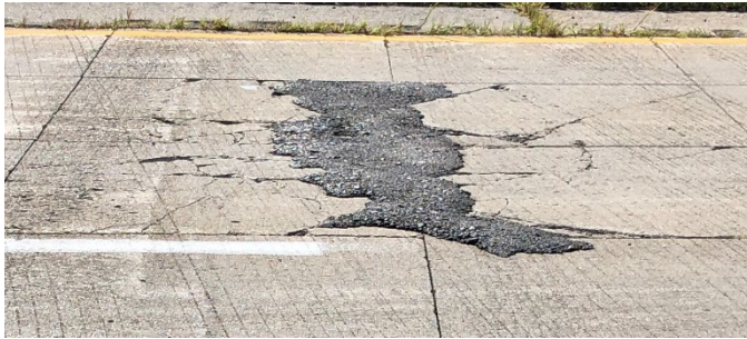
e) Shattered slabs in passing lane
