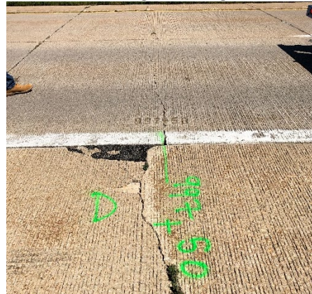
d) Mid-panel trans. cracking (997+50)
