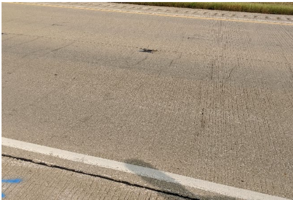
c) Y-cracking and cluster cracking (248+40 EB)
