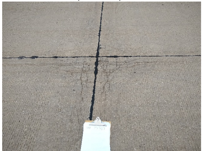
f) Corner distress in DL (25+340 SB)
