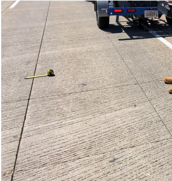
a) Long. jt in driving lane
