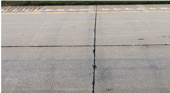
c) Longitudinal joint faulting (Section WB-2)
