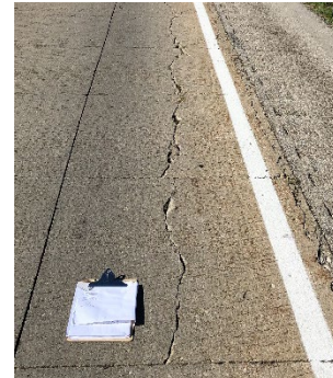
h) Severe long. cracking & corner breaks in OWP
