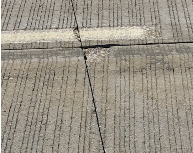
a) Corner distress on leave joint left panel in driving lane
