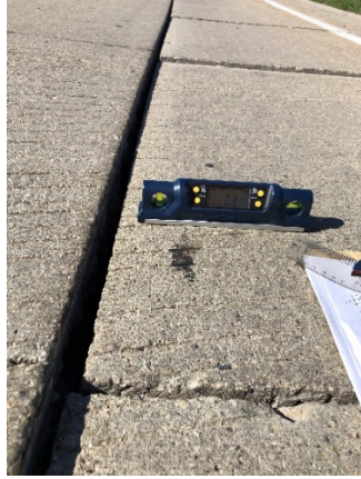
a) Severe long. faulting along OWP DL long. jt.
