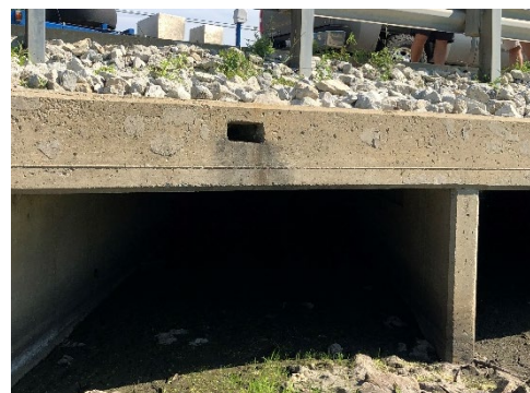
f) Culvert causing cracking in PCC (72+00 EB)
