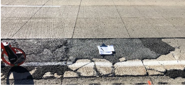
a) Shattered slabs with HMA patching (2+27 SB)
