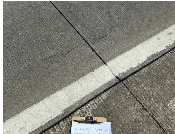
d) Longitudinal crack over dowel in OWP (2+140 EB)
