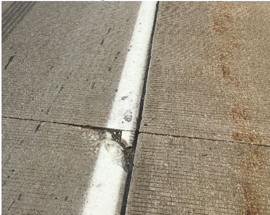
c) Corner distress along approach joint in DL (180+45 NB)
