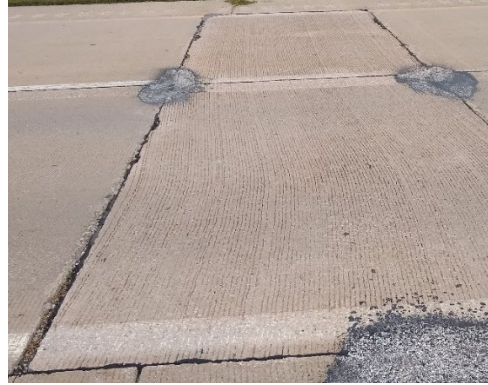
b) Old FDR with excessively wide joints and HMA or spray injection patches (28+615 SB)
