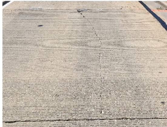
d) Long. cracking spanning two panels (57+25 WB)
