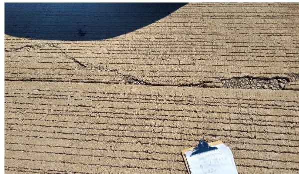
d) Severe joint damage in DL and Shoulder - Approach (3299+68 WB)
