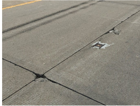
b) Corner distress in DL and Reflector damage (1+330 EB)
