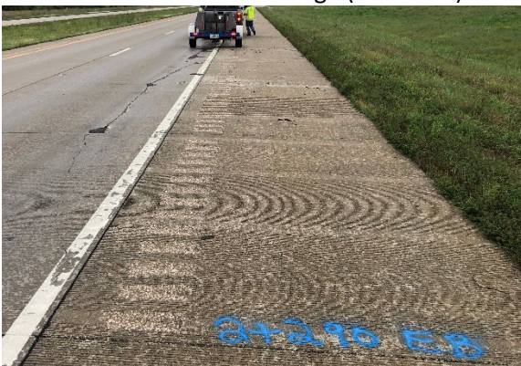
e) Edge failure due to lack of support (2+290 EB)
