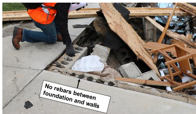
Figure 2.4. Residential rated DOD 8 due to unreinforced masonry foundation walls.
