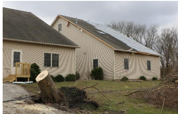
(b) damage survey image
