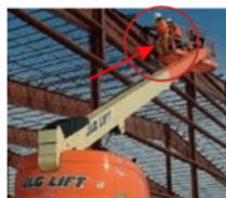
Observed one of the ironworkers standing on midrail when I arrived.
