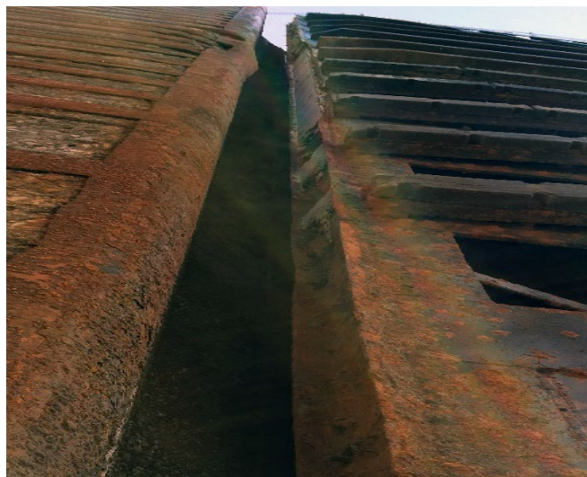
Figure 2.11. Meldahl miter gate, with section of quoin block missing.
