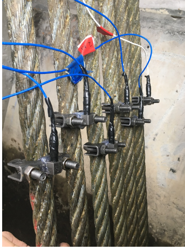
Figure 6.8 Accelerometers on cables at The Dalles.
