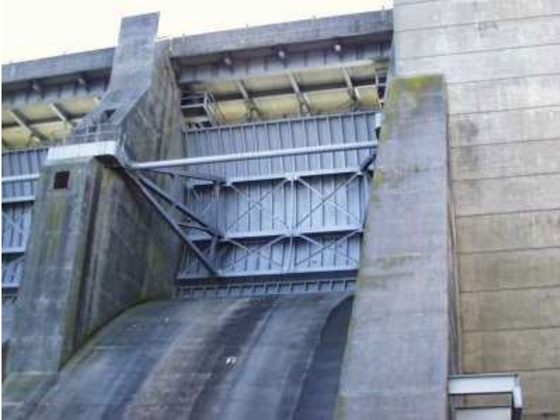
Figure 1.6. Typical Tainter gate on a dam. (U.S. Army Corps of Engineers n.d.).
