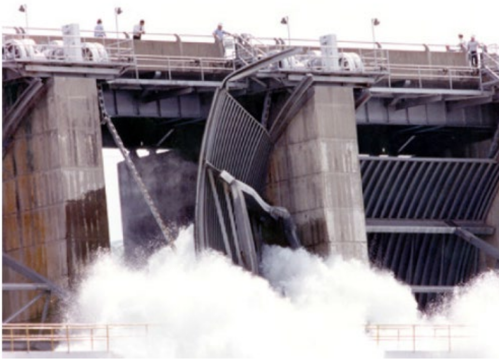
Figure 2.23. Failure of Folsom dam Tainter gate due to excessive trunnion friction, uneven hoisting, and buckled strut arms (U.S. Army Corps of Engineers n.d.).
