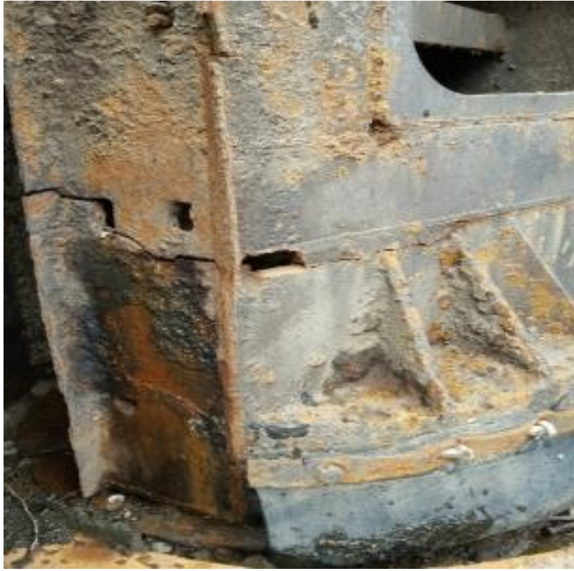
Figure 2.12. Pintle region of Meldahl miter gate with extensive cracking due to lack of quoin contact.
