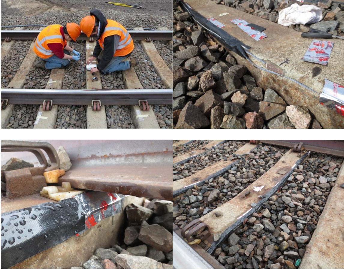
Figure 2.5: Images of cross-ties instrumented with concrete surface strain gauges at a heavy-haul freight railroad field experimentation location.
