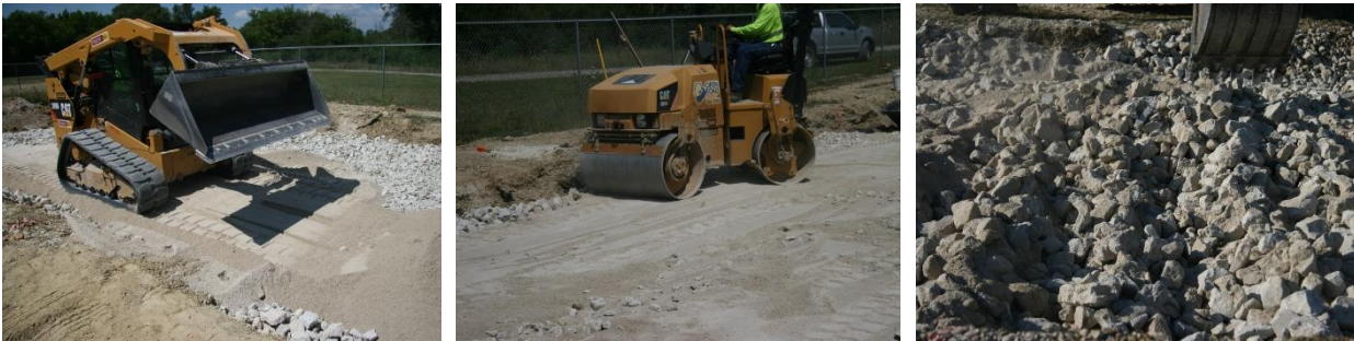
Construction of the first lift in the two-lift PCR/QB1 test section (C1S1)
