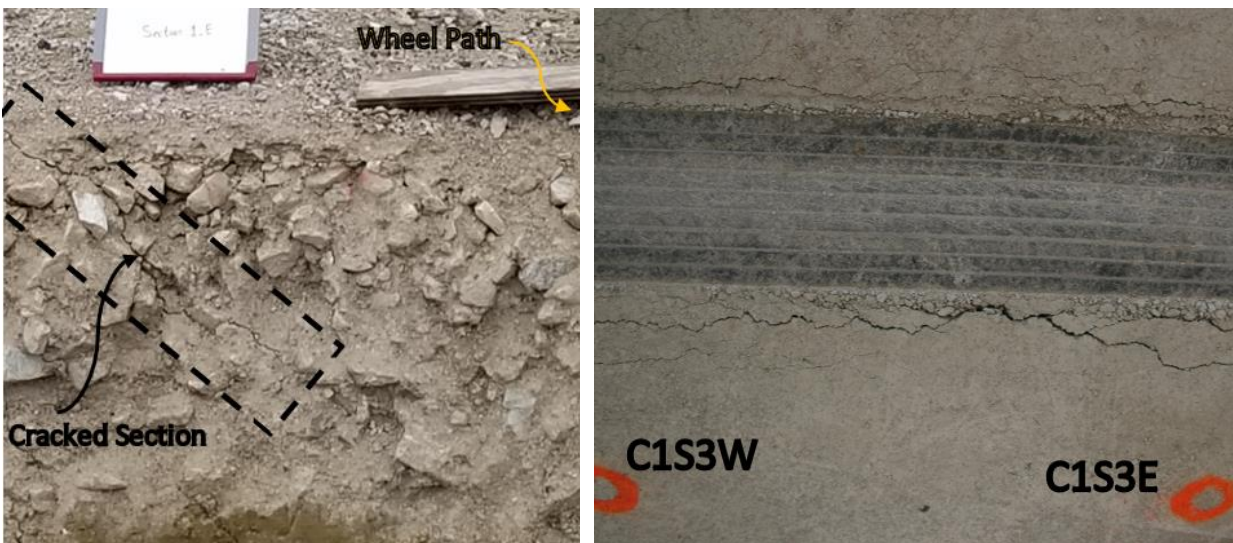
Cracking in C1S1E (PCR/QB1 – 2 Lifts)
