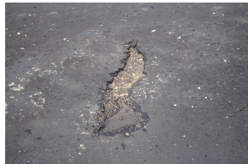
(b) Pothole associated with chip loss
