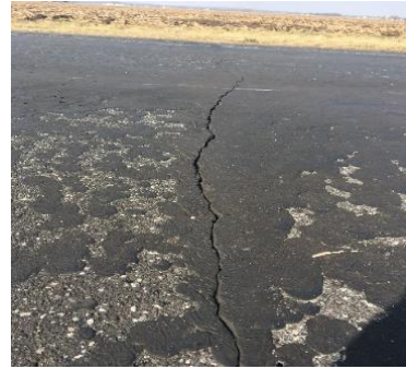
(b) Transverse cracks
