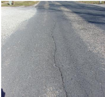
(c) Longitudinal cracks
