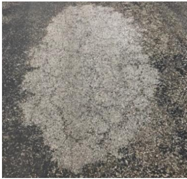
(a) Patch deterioration with cracks
