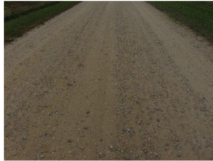
Figure 16. Insufficient gravel on gravel road.
