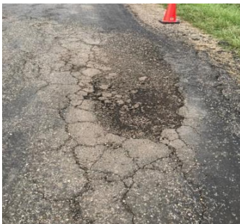
(a) Pothole associated with cracks
