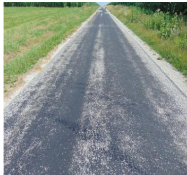
Figure 10. Bleeding of asphalt binder in seal-coated road.
