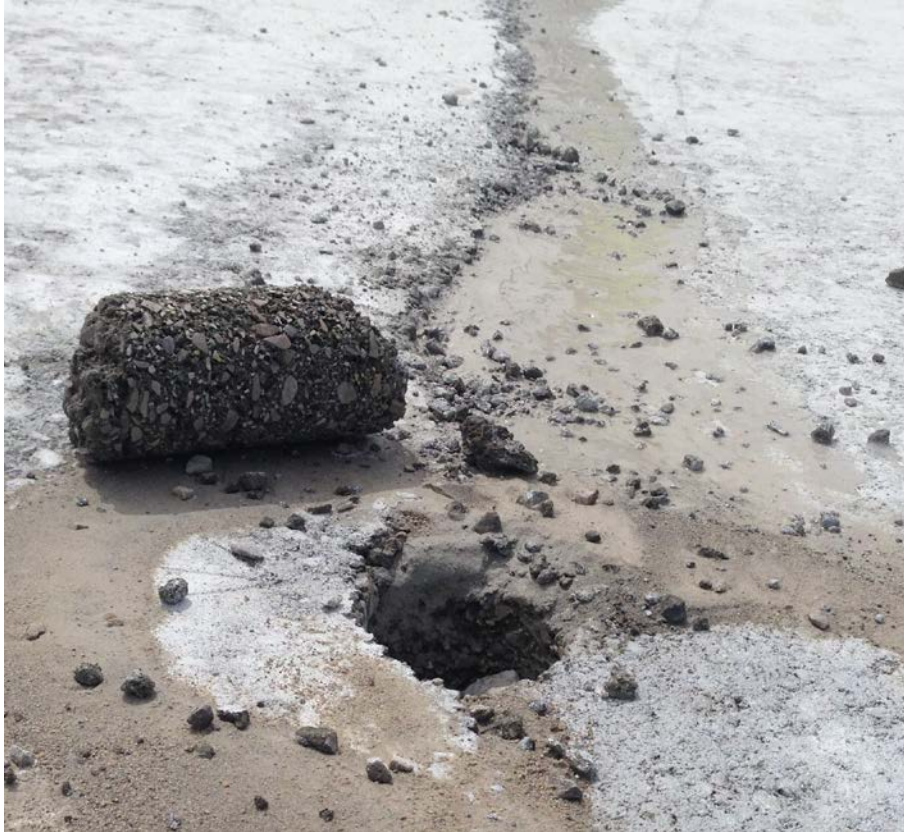
Figure 24. Core from cold joint.
