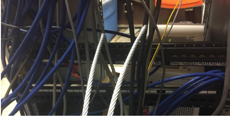
Figure K5. Patch Panels for Ethernet Connection.
