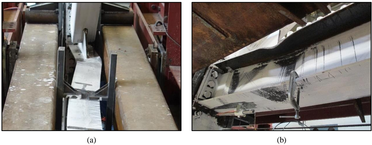
Figure 4.10 – R = 3 chevron frame Level 2 beam crushing and buckling while attempting to exercise Story 1.
