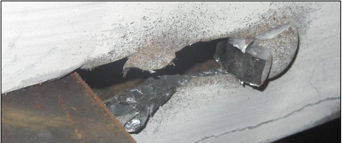
Figure 4.17 – Story 1 South brace lower connection HSS slot, R = 3 chevron CBF Phase IV. The effective thickness of the slot has increased to five times its original thickness due to bearing on the gusset plate.
