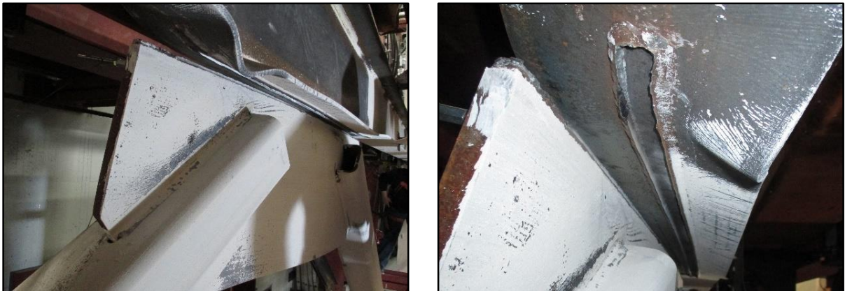
Figure 4.30 – Level 2 beam bottom beam-gusset weld fracture, R = 3.25 split-x OCBF.
