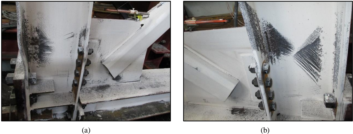
Figure 4.31 – Lower Story 2 column (Level 1) plastic hinging, R = 3.25 split-x OCBF: (a) South column; and (b) North column.
